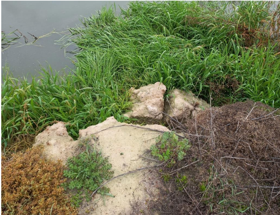
Photo B-4: Evidence of internal pond banks crumbling
