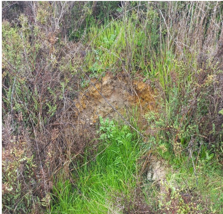
Photo B-1: Vegetation and crumbling of pond outer bank
