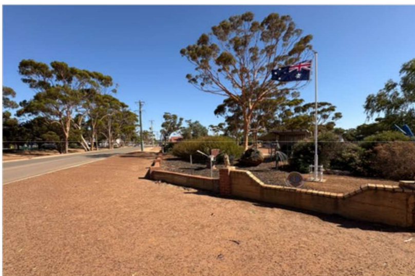
Figure 3: Existing Western Power Overhead WPC services along McPherson St.
